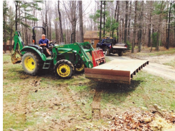
Getting rid of some of the demolished back section of the store
